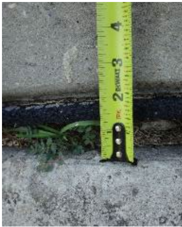
Gap at walk leading to Unit 1825.
