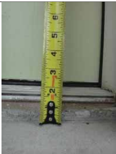
Threshold and change in level at primary entrance threshold exterior side, 1212 Rev. John Raphael Jr. Way.
